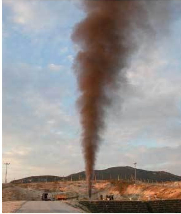
DEPA purged the valve station at the entrance of the border metering station with gas after pigging in order to dispose of any remaining powder and prevent rapid clogging of the cartridge filters, venting large amounts of black powder in the process (Fig. 5).
