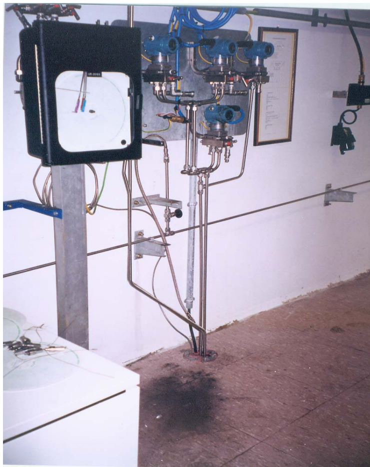
Figure 2. Instrumentation of a gas metering line. Black powder removed from only one pressure transmitter is appearing on the floor.
