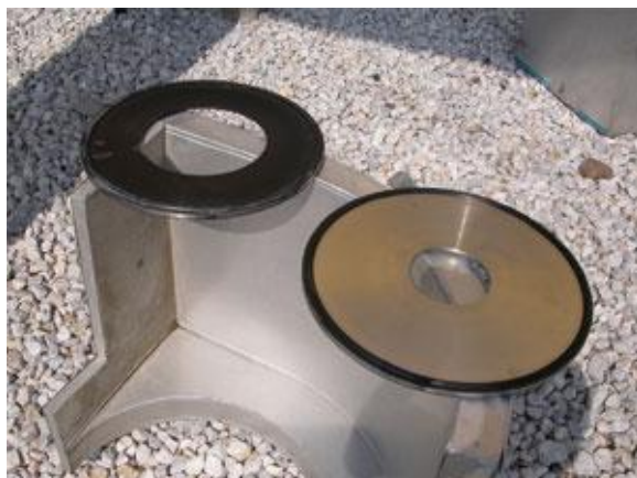
Black powder thoroughly coated the orifice plate shown on the left of this photograph. A clean orifice plate provides contrast (Fig. 2).
