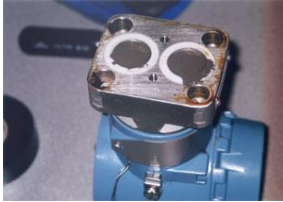
Black powder has almost completely blocked this pressure transmitter (Fig. 5).
