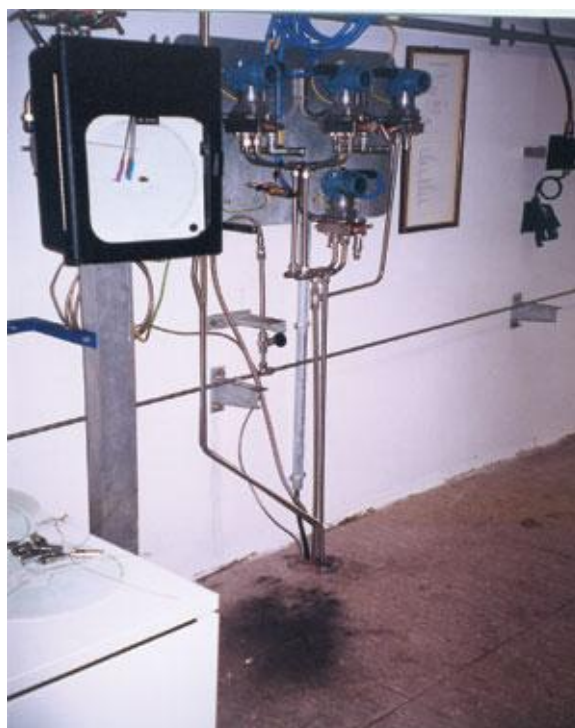
Black powder from just one gas pressure transmitter lies on the floor beneath the transmitter assembly and metering instrumentation (Fig. 3).
